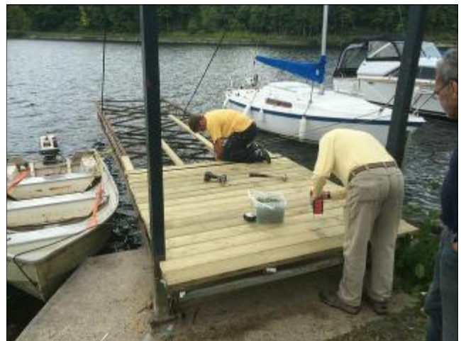
The volunteer dock repair crew spent a weekend upgrading and repairing finger docks so that they are as good as new.
